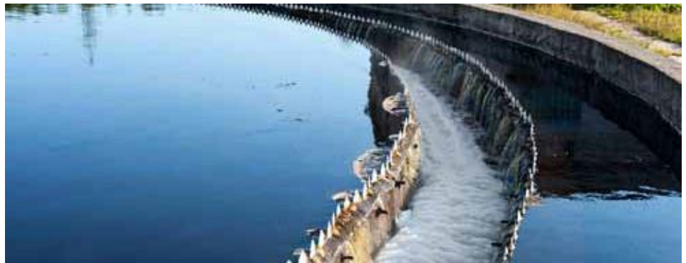
After an 2800 gallon sodium hypochlorite storage tank ruptured and began leaking at the South Berwick wastewater treatment plant, the plant switched to calcium hypochlorite for its final disinfection operations.
