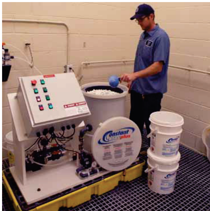
Loading Constant Chlor® cal hypo briquettes into the hopper of Little Egg Harbor MUA's Arch Constant Chlor™ MC4-50. The unit is designed to supply up to 50 lbs of AvCl/day.
