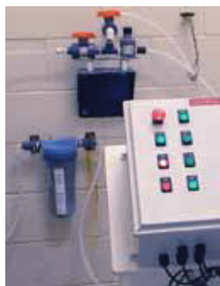
Little Egg Harbor MUA's installation of a small filtration system (blue unit on wall, lower left) provides a solution for preventing scaling problems that is now used by Arch at most of its new installations.
