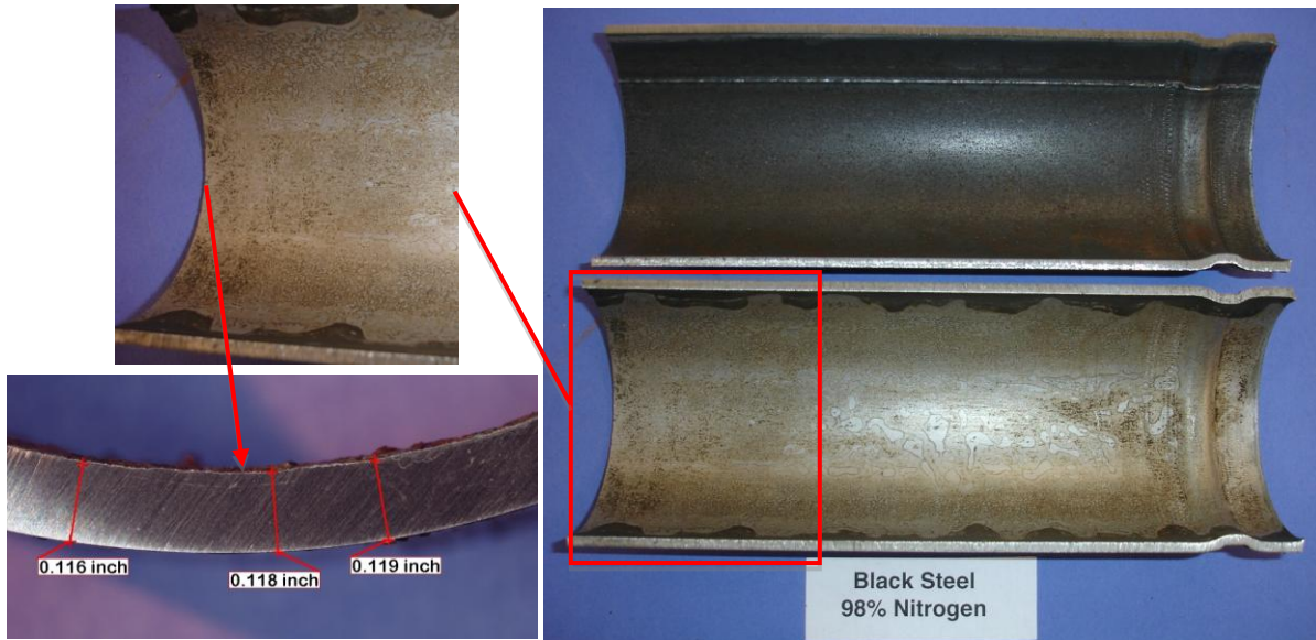
Figure 4. Black steel piping after 498 days exposure while half-filled with water and 98% nitrogen supervision. Note uniform appearance of pipe wall and absence of any localized pits.
